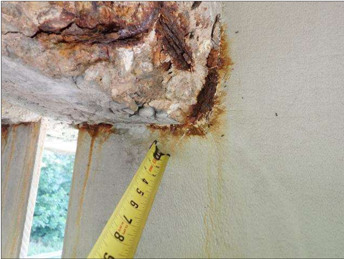
Span 3 Beam 1: at bent 2, web adjacent to diaphragm, painted over section loss (1/2 inch average remaining x 10 inch x 5 inch) with corrosion reinitiated
