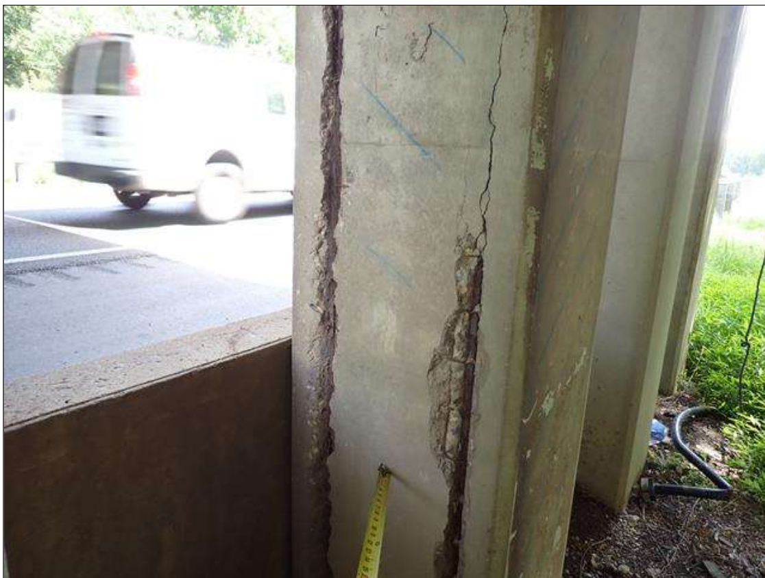
Bent 1 Pile 5: (PAR) west, east and south faces, spalls/delaminations (up to full height x 17 inch x 1 inch deep) with cracks (up to 1/8 inch) and exposed H-pile flanges; flanges have rust scale
