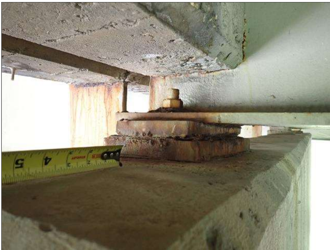
Span 1 Beam 2 - Far Bearing 2: SPAN 1 FAR BEARING HAS RUST SCALE/PACK RUST
