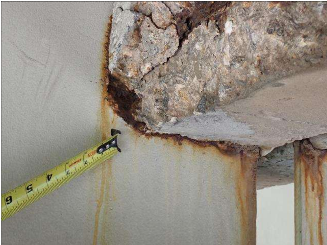
Span 3 Beam 2: at bent 2, web adjacent to diaphragm, corrosion with section loss (1/2 inch average remaining x 9 inch x 2 inch)
