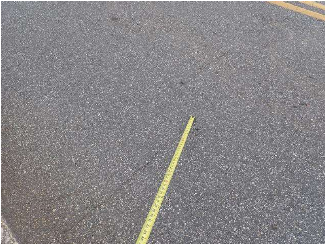
Span 2 Wearing Surface: WEARING SURFACE HAS SCATTERED MAP/TRANSVERSE AND LONGITUDINAL CRACKS [up to 12 feet x UP TO 1/8 INCH]
