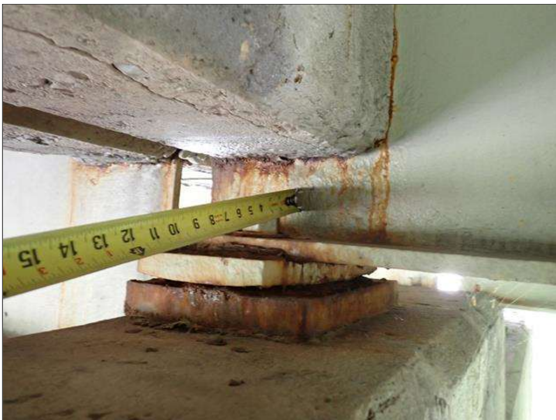
Span 1 Beam 4: (PAR) at bent 1, web adjacent to diaphragm, painted over section loss (3/8 inch average remaining x 9 inch x 4 inch) with corrosion reinitiated
