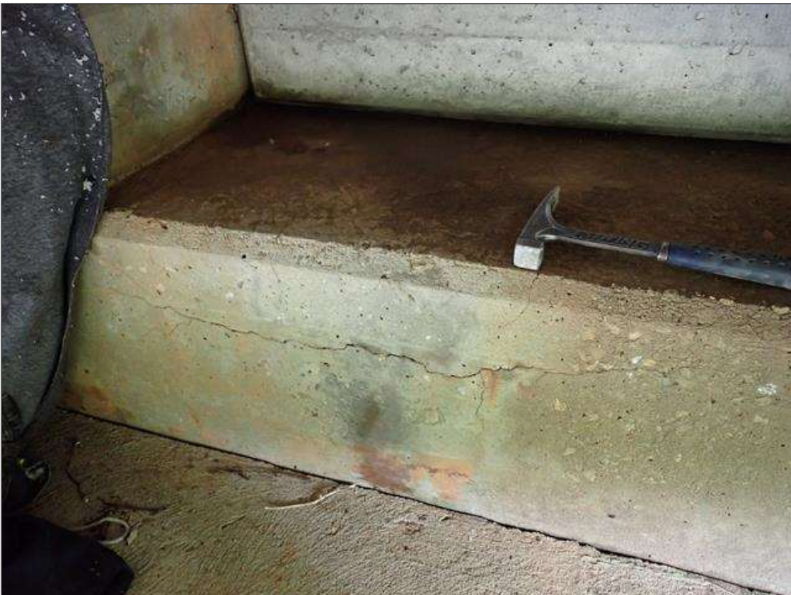
End Bent 1 Cap 1: (PAR) in bays 1 and 4, delaminations (up to 6 feet x 10 inch) with cracks (up to 1/4 inch wide) and rust stains
