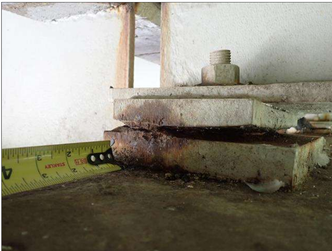
Span 4 Beam 4 - Near Bearing 4: SPAN 4 NEAR BEARING HAS PACK RUST.
