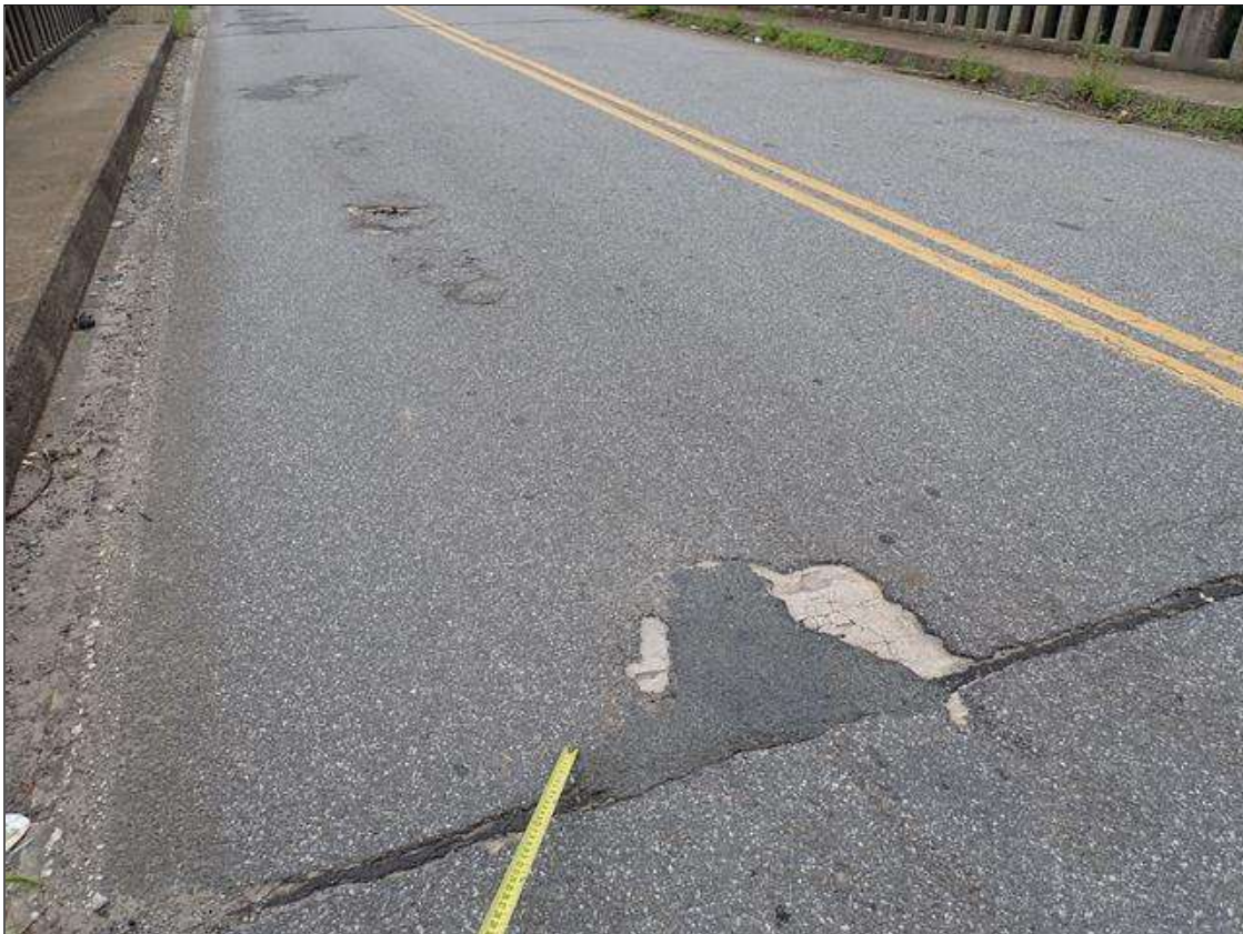
Span 3 Wearing Surface: (PAR) throughout wearing surface, areas of delaminations (up to 3 feet x 2 feet) with cracks (up to 1/4 inch); northbound lane, spalls (up to 27 inch x 2 feet x full depth)
