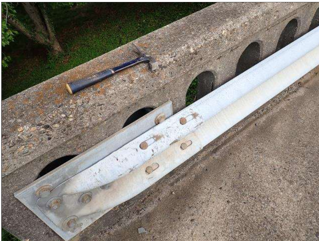
(PAR) northwest guardrail attachment, improper lap
