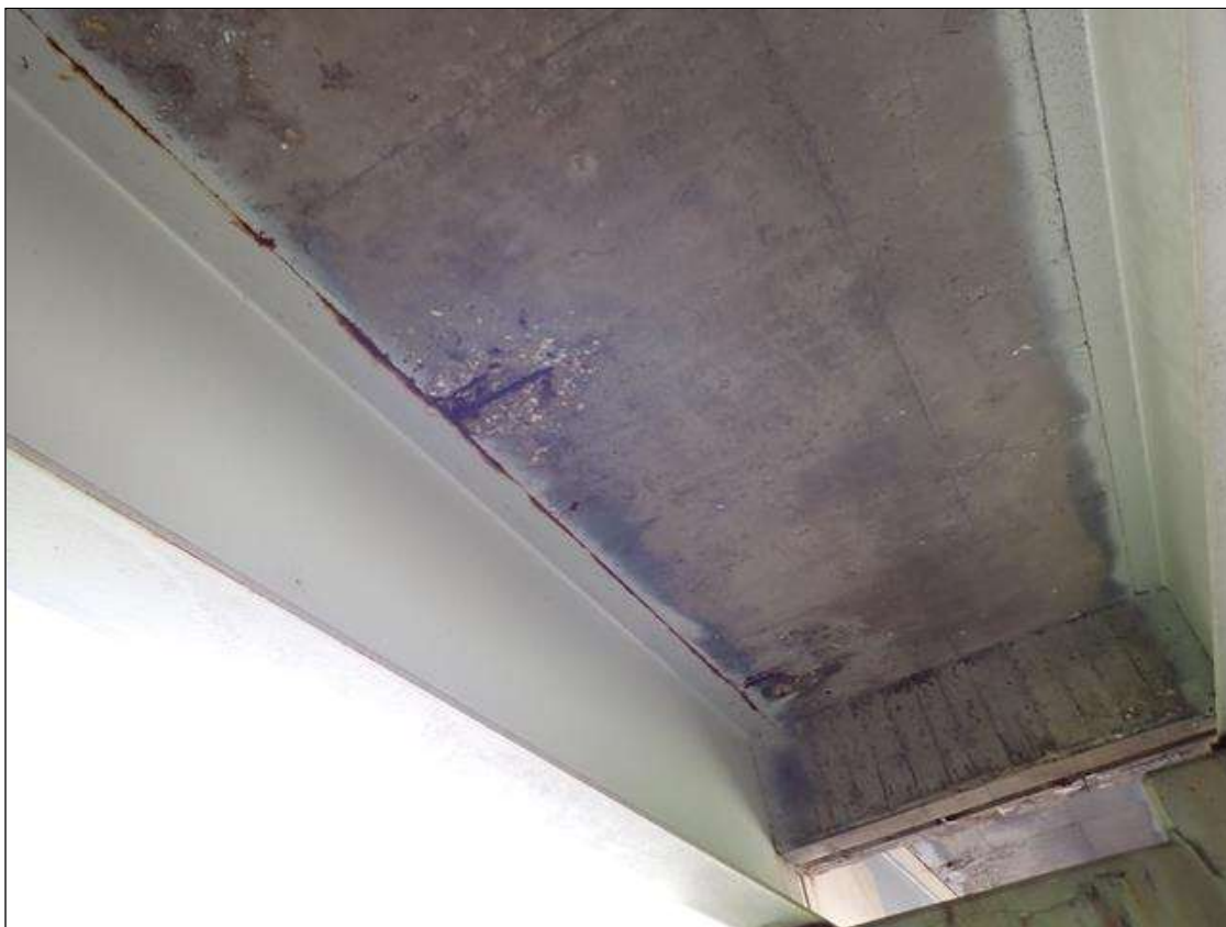
Span 1 Deck: (PAR) underside of bays 1 and 4, and both overhangs at bent 1, spalls/delaminations (up to 2.5 feet x 15 inch x 2.5 inches deep) with exposed rusted rebar; rebar has approximately 10 percent section loss
