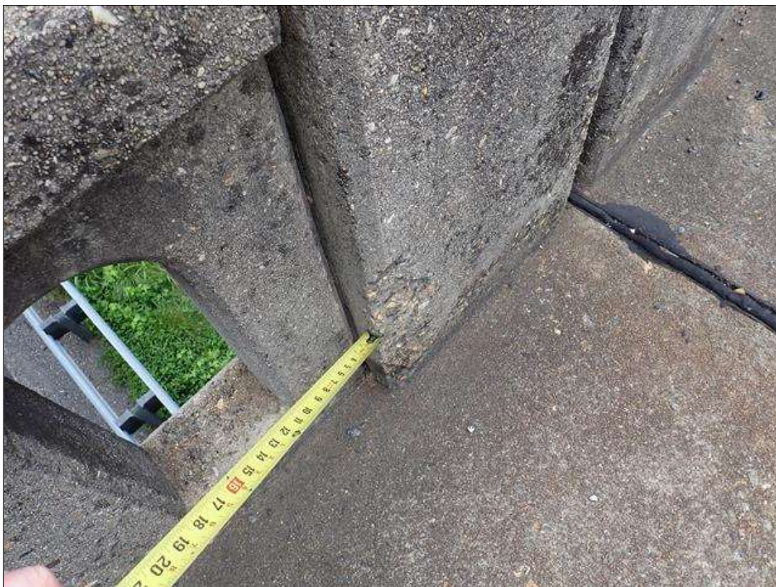
Span 2 Left Bridge Rail: along the length of the rail, spalls (up to 14 inch x 4 inch x 1 inch deep), some with exposed rusted rebar
