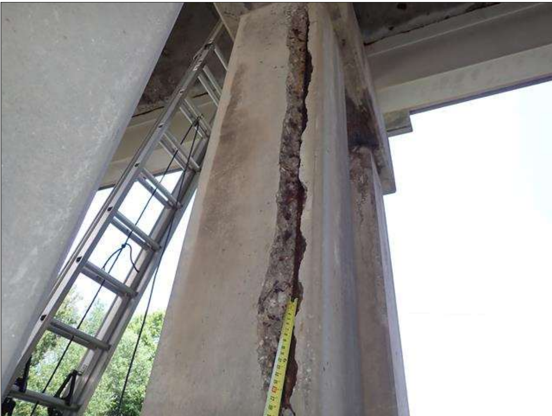
Bent 2 Pile 6: (PAR) west and east faces, spalls/delaminations (up to full height x 8 inch x 3 inches deep) with cracks (up to 1/4 inch) with efflorescence; H-pile flange exposed with rust scale
