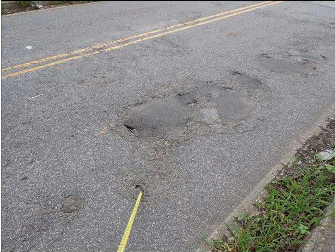
Span 1 Wearing Surface: (PAR) throughout wearing surface, areas of delaminations (up to 3.5 foot diameter) with cracks (up to 1/4 inch); both travel lanes, spalls/failed patches (up to 7 feet x 4 feet x full depth)
