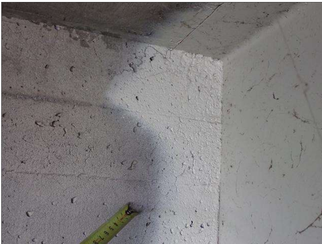
End Bent 1 Abutment: HAIRLINE MAP CRACKING AT RANDOM THROUGHOUT.
