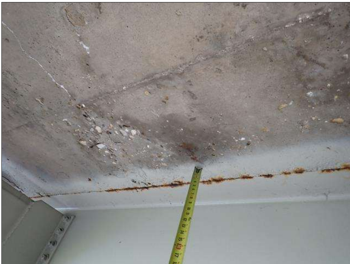
Span 1 Deck: (PAR) BOTTOM OF DECK UP TO 1/32 INCH MAP CRACKING AT RANDOM THROUGHOUT SOME WITH EFFLORESCENCE AND RUST STAINS
