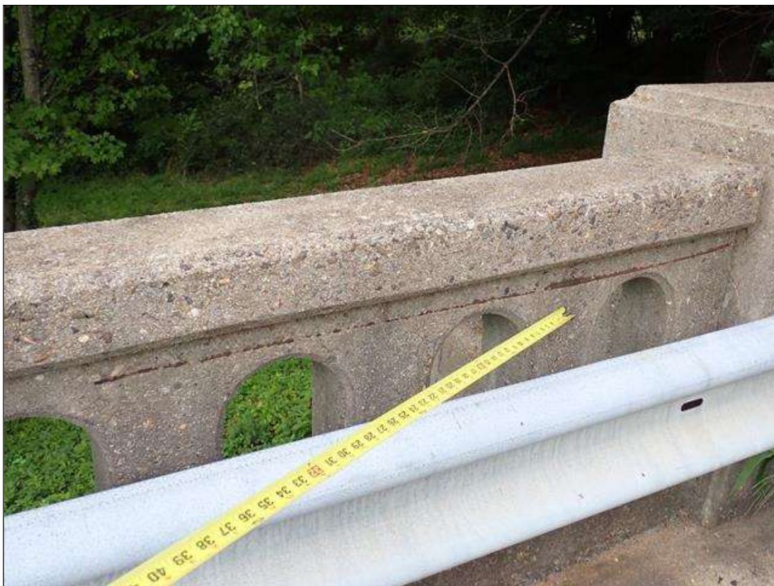
Span 4 Left Bridge Rail: top of rail, at end bent 2, shallow rebar
