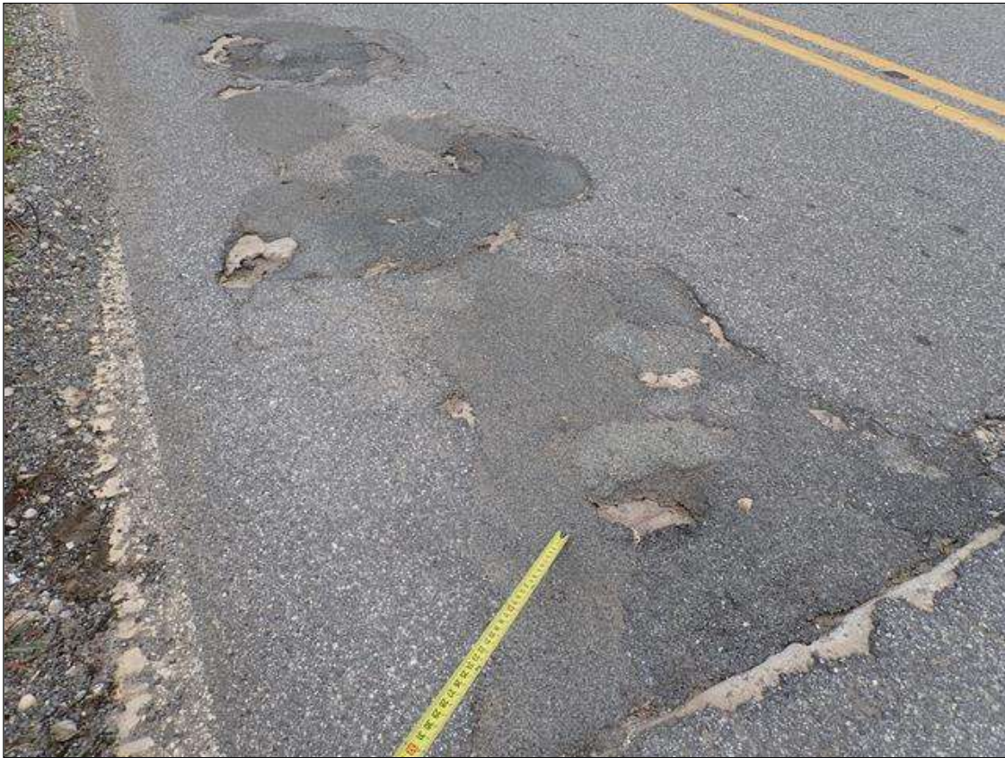
Span 2 Deck: (PAR) throughout top of deck, at areas of missing asphalt, spalls/delaminations (up to 28 inch x 1 foot x 1.5 inch deep), some with exposed rusted rebar
