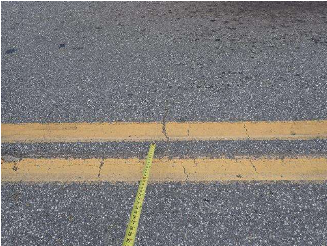
Span 4 Wearing Surface: SPAN 4 WEARING SURFACE HAS SCATTERED TRANSVERSE AND LONGITUDINAL CRACKS [up to 5 feet x UP TO 1/4 INCH]
