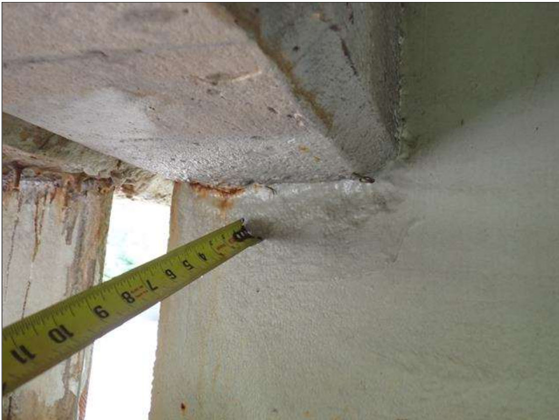
Span 1 Beam 5: at bent 1, web adjacent to diaphragm, painted over section loss (1/2 inch average remaining x 10 inch x 2 inch) with corrosion reinitiated
