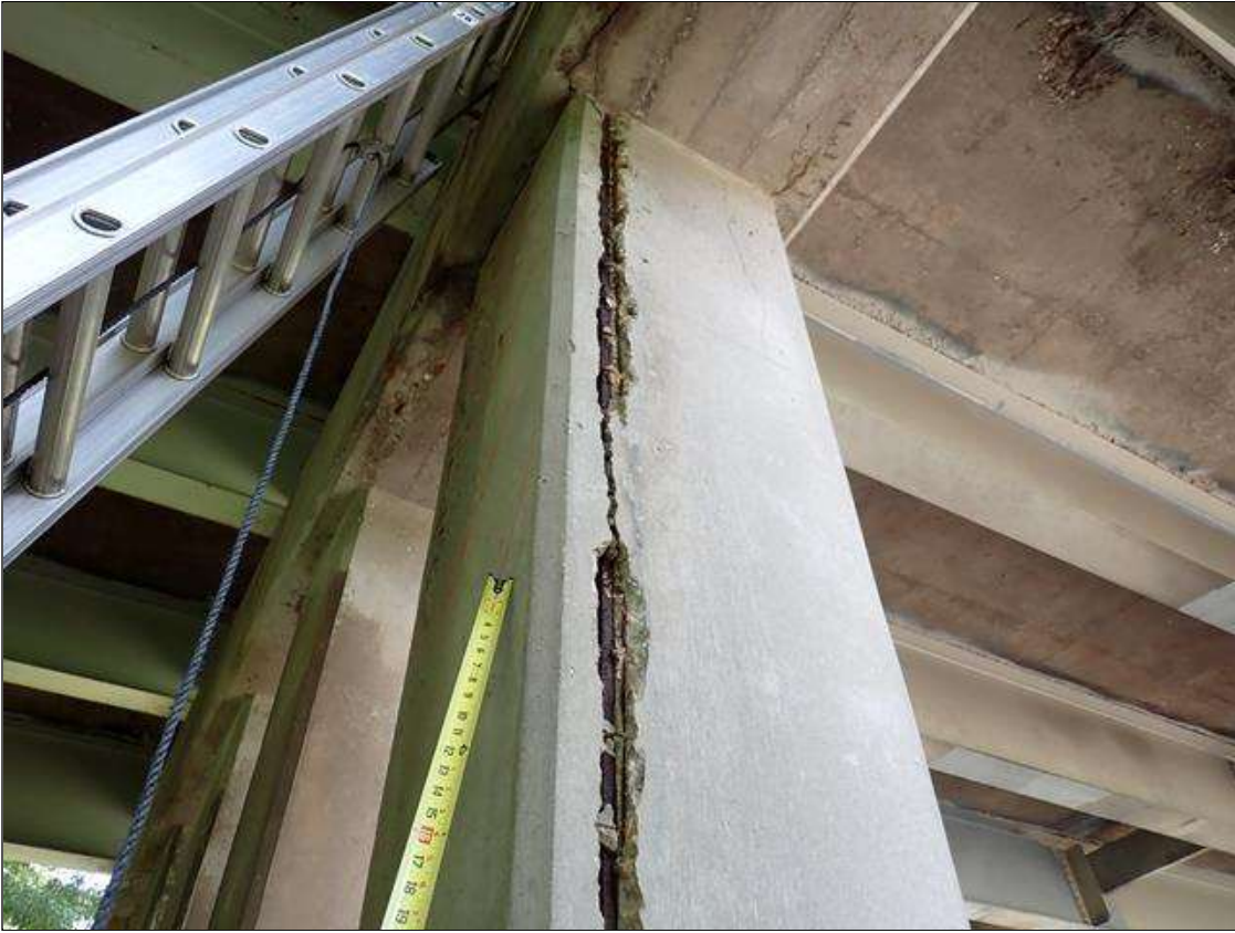
Bent 1 Pile 6: (PAR) west, east and south faces, spalls/delaminations (up to 11 feet x 18 inch x 1 inch deep) with cracks (up to 1/4 inch) and exposed H-pile flanges; flanges have rust scale
