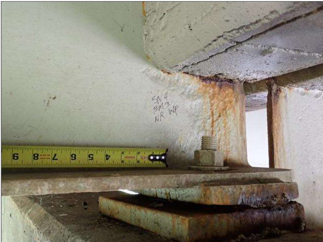
Span 4 Beam 3: (PAR) at bent 3, painted over section loss: web adjacent to diaphragm (5/16 inch average remaining x 9 inch x 2 inch), lower web (7/16 inch average remaining x 6 inch x 1 inch) with corrosion reinitiated
