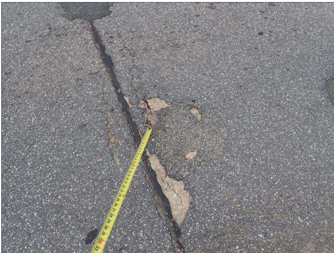
Span 1 Deck: (PAR) throughout top of deck, at areas of missing asphalt, spalls/delaminations (up to 2 foot x 1 foot x 1.5 inch deep), some with exposed rusted rebar
