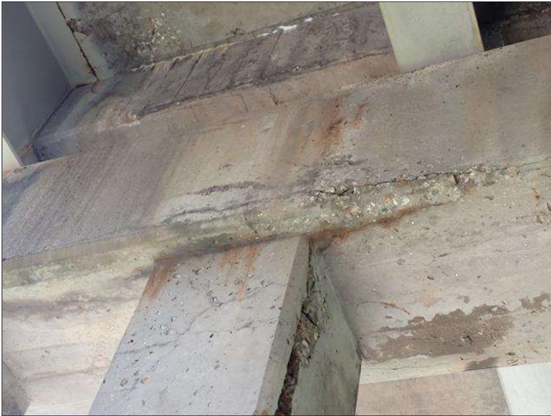
Bent 2 Cap 1: (PAR) south and north faces, spalls/delaminations (up to 6 feet x 8 inch x 1 inch deep) with cracks (up to 1/8 inch), some with rust stains
