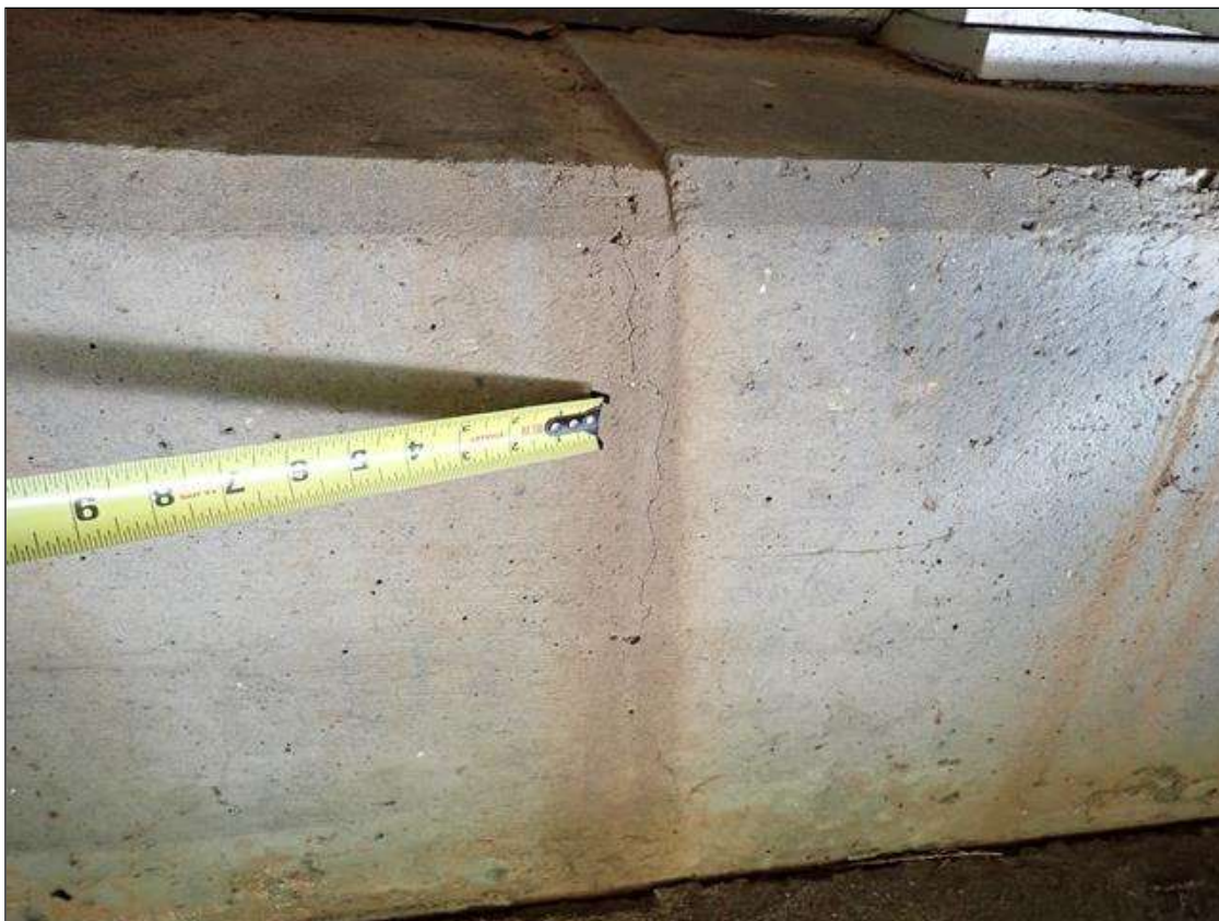
End Bent 2 Cap 1: up to full height x UP TO 1/64 INCH VERTICAL CRACKS, AT RANDOM, some wraparound
