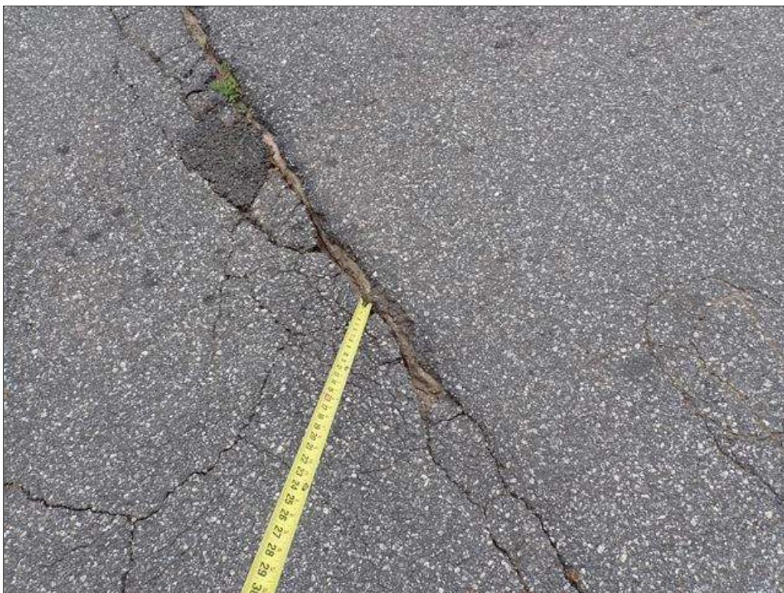
Span 4 Deck: top of deck, at end bent 2, at areas of missing wearing surface, edge spalls (up to 1.5 feet x 2 inch x 1 inch deep)
