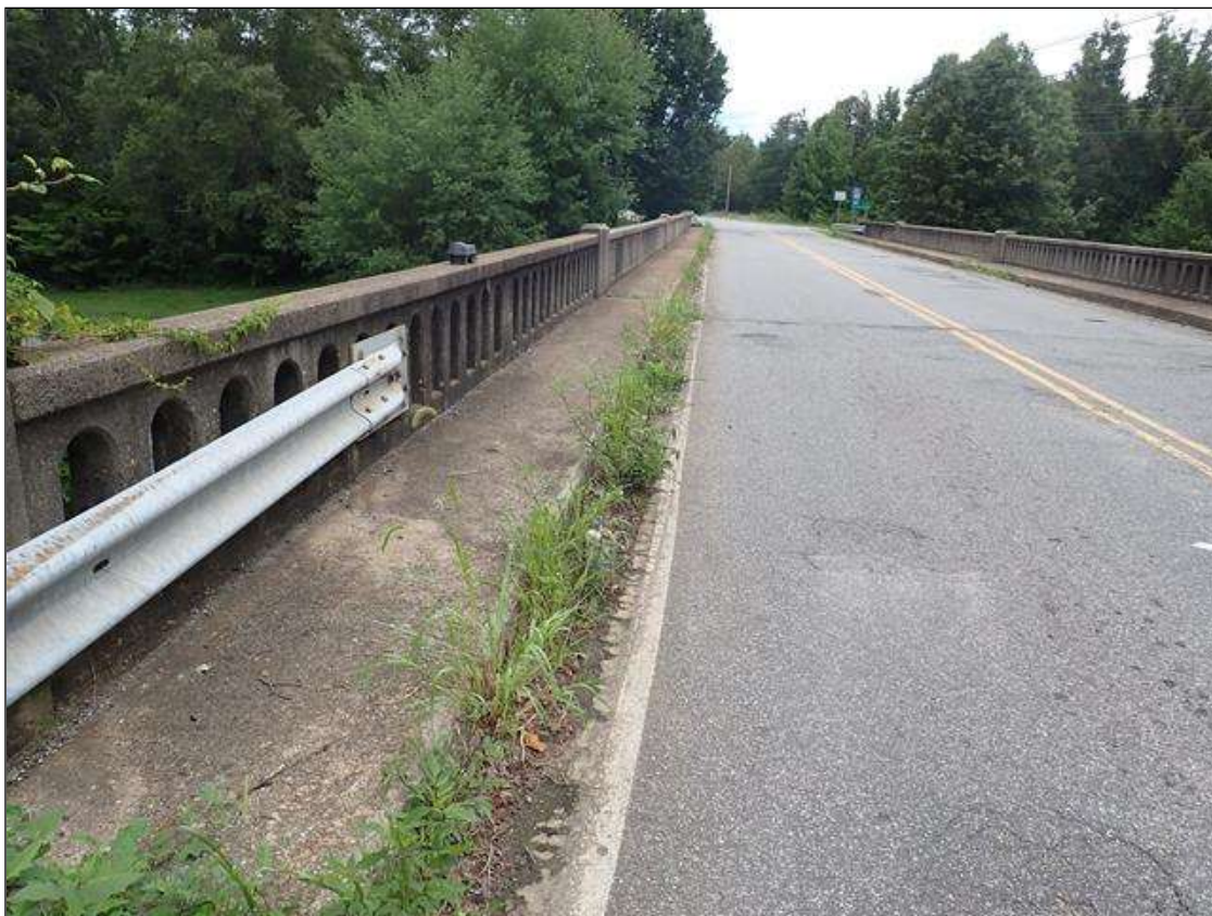
along the curblines, debris accumulation (up to 15 inches high x 3 inches wide) with vegetation, obstructing deck drainage
