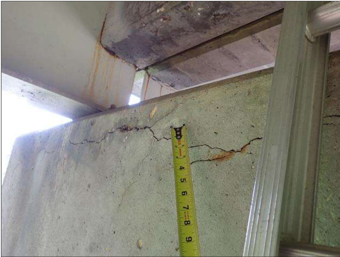
Bent 3 Cap 1: (PAR) south and north faces, below all bays, spalls/delaminations (up to 7 feet x 2 feet x 1/2 inch deep) with cracks (up to 1/16 inch) and rust stains
