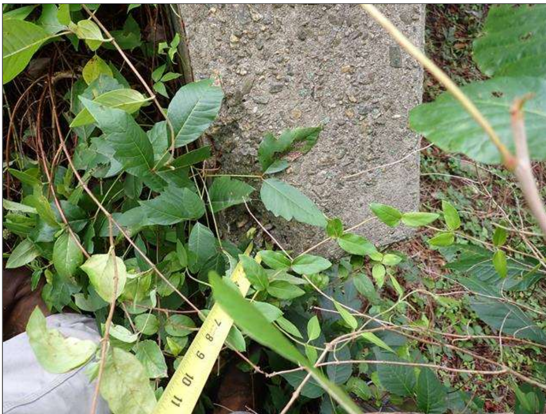
southeast wingwall, at end, spall (9 inch x 6 inch x 2 inch deep)
