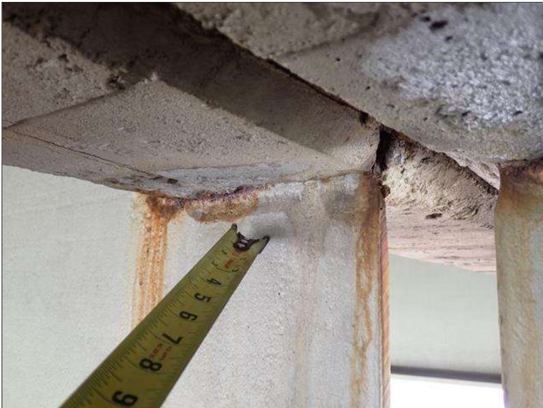
Span 2 Beam 3: (PAR) at bent 2, web adjacent to diaphragm, painted over section loss (3/8 inch average remaining x 9 inch x 2 inch), with adjacent pitting (up to 1/8 inch deep), with corrosion reinitiated
