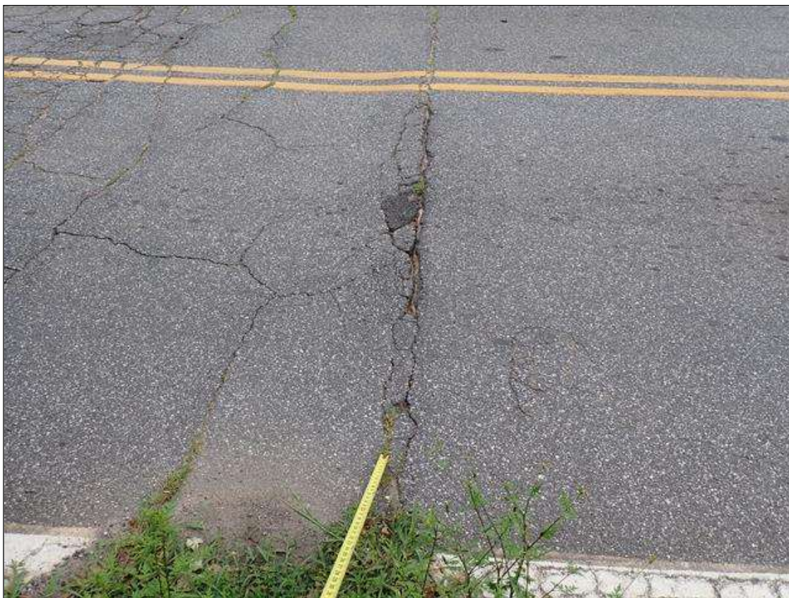
Span 4 Wearing Surface: over end bent 2, transverse crack (up to 1 inch wide x full width of roadway) with edge spalls (up to 3 inch wide x 1.5 inch deep) and vegetation
