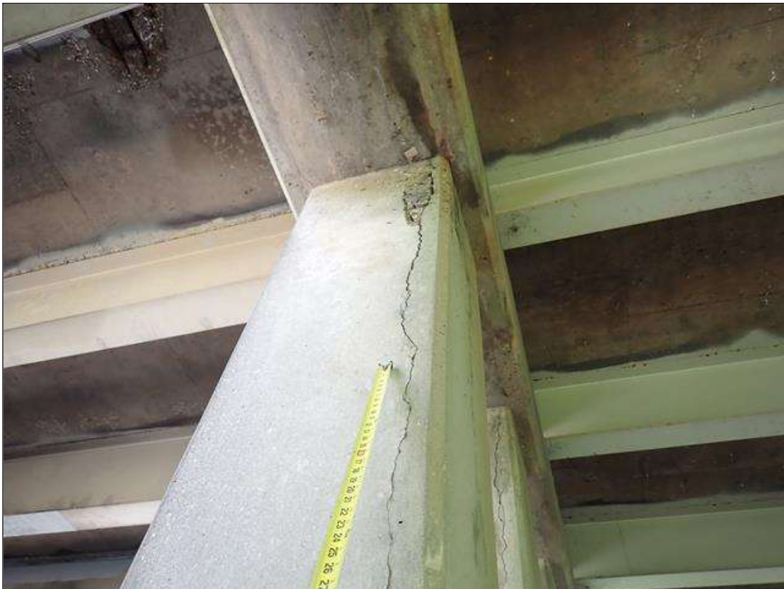
Bent 1 Pile 2: west, east and south faces, near cap, spalls/delaminations (up to 5.5 feet x 8 inch x 1 inch deep) with cracks (up to 3/16 inch)
