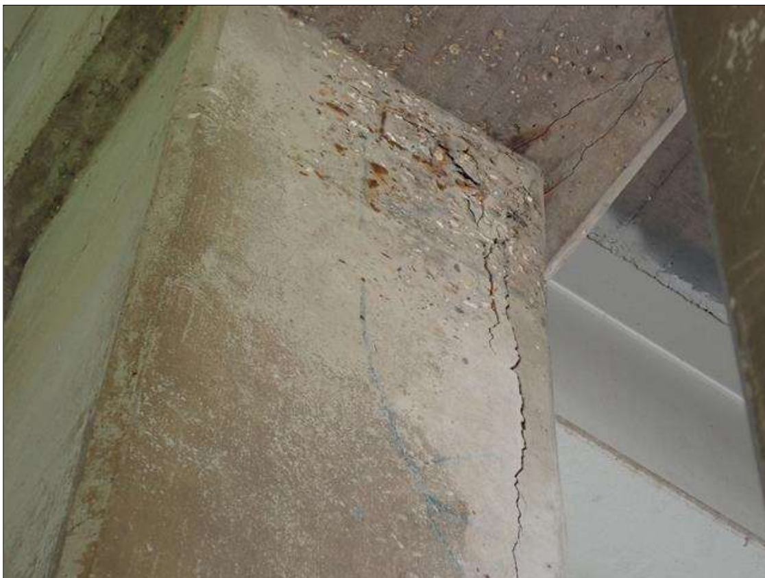
Bent 3 Pile 5: (PAR) southwest and southeast corners, at cap, delaminations (up to 3.5 feet x 1 foot) with cracks (up to 1/8 inch) and rust stains
