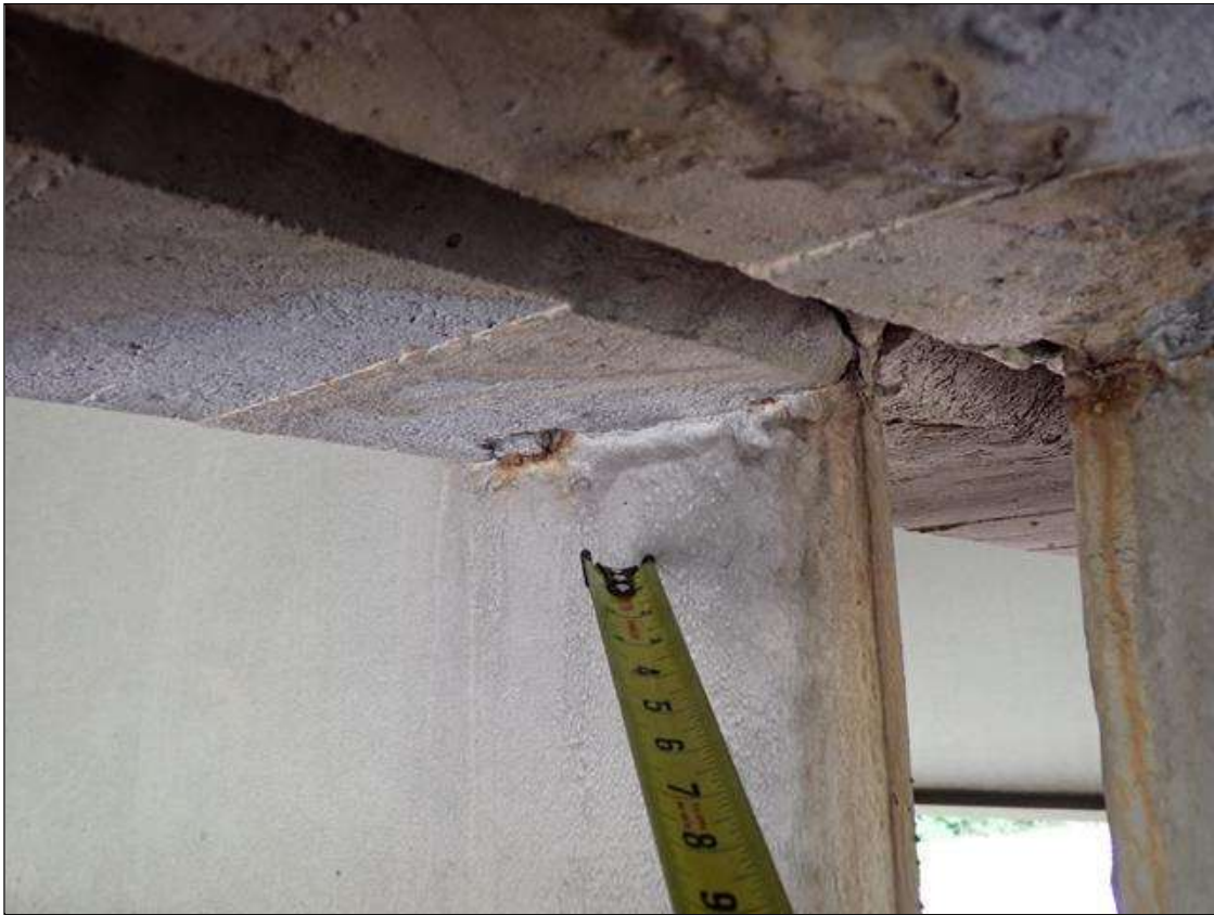
Span 2 Beam 4: (PAR) at bent 2, web adjacent to diaphragm, painted over section loss (3/8 inch average remaining x 8 inch x 2 inch), with adjacent pitting (up to 1/8 inch deep), with corrosion reinitiated
