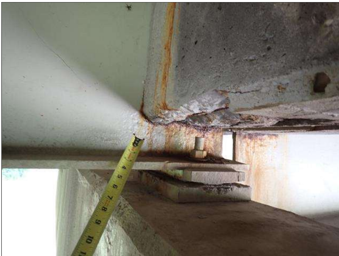
Span 1 Beam 3: (PAR) at bent 1, web adjacent to diaphragm, painted over section loss (3/8 inch average remaining x 10 inch x 2 inch) with corrosion reinitiated
