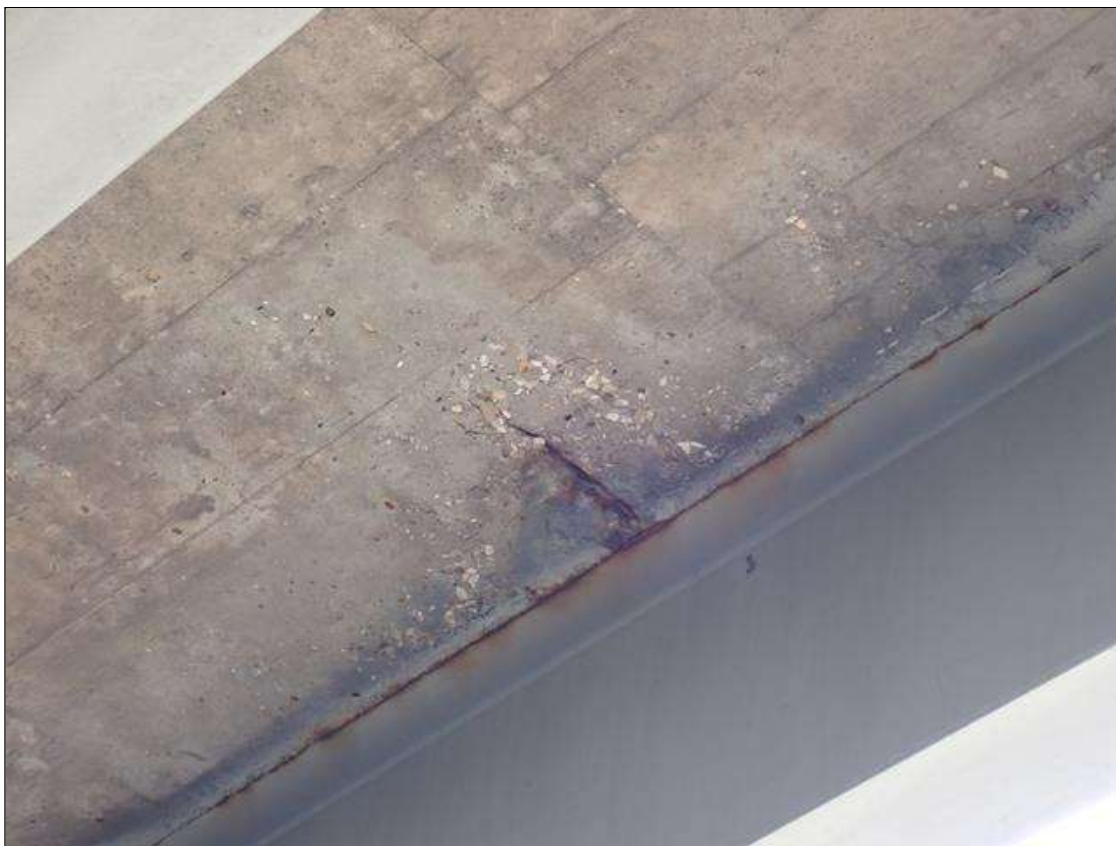
Span 3 Deck: (PAR) underside of bays 1 and 4, spalls/delaminations (up to 2 foot diameter x 2.5 inches deep) with exposed rusted rebar; rebar has approximately 5 percent section loss
