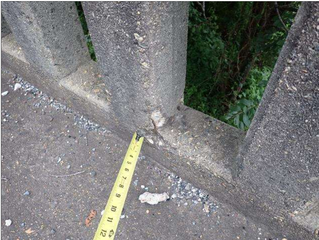
Span 4 Right Bridge Rail: RIGHT RAIL HAS SCATTERED AREAS THAT ARE CRACK/SPALL [up to 18 inch x 2 inch x 1 inch deep] AND DELAMINATED WITH REBAR EXPOSED [no section loss]
