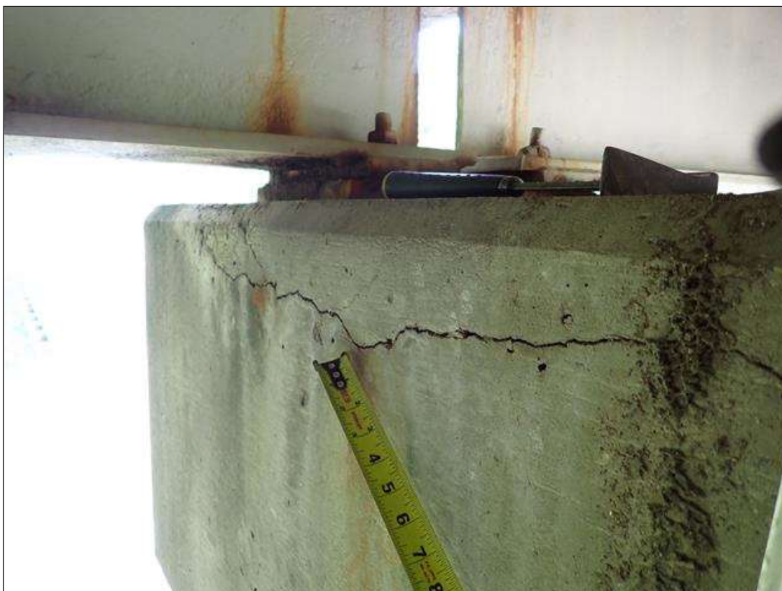
Bent 1 Cap 1: (PAR) south and north faces, below all bays, delaminations (up to 5.5 feet x 6 inch) with cracks (up to 1/8 inch) and rust stains
