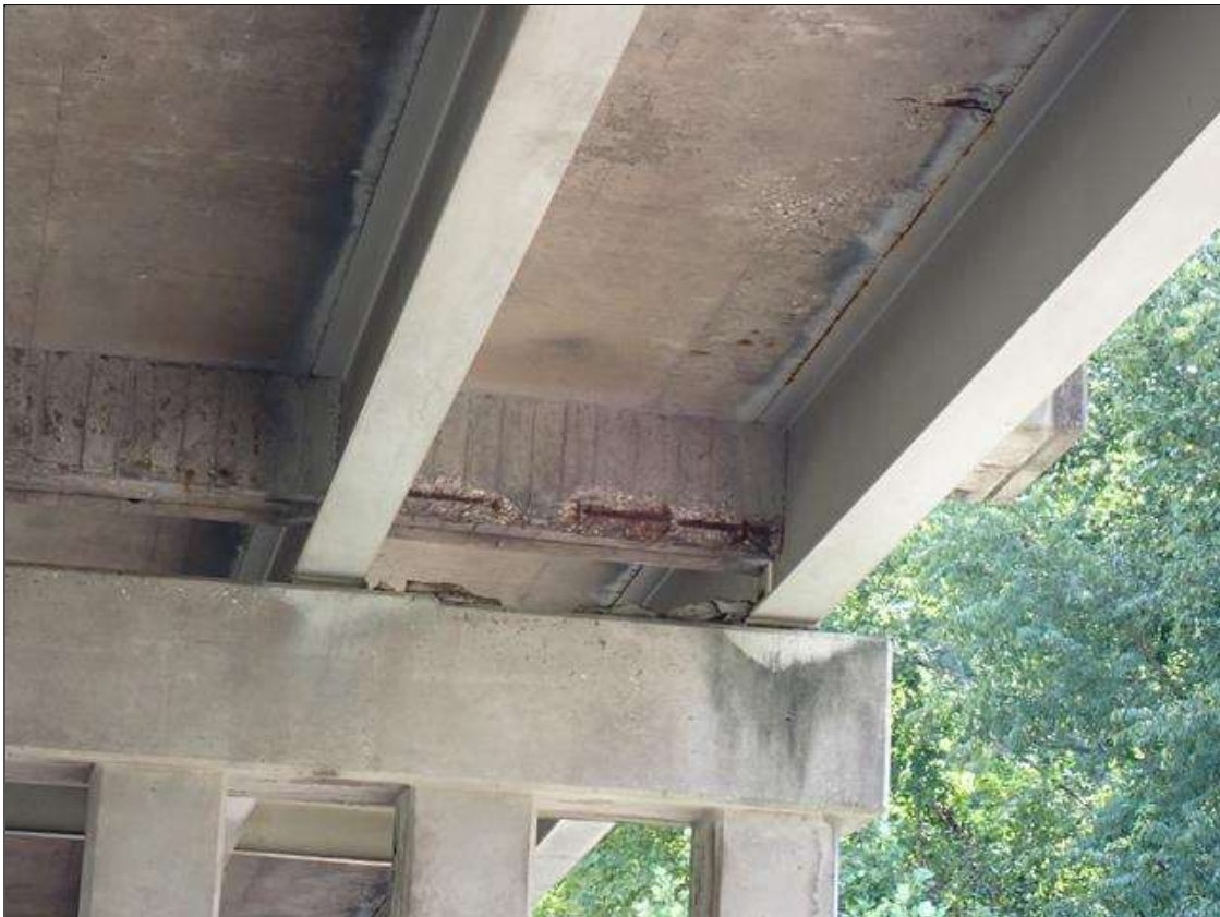
Span 3 Deck: at bent 2, end diaphragms in all bays and overhangs, spalls/delaminations (up to full bay width x 8 inch x 2 inches) with exposed rusted rebar and cracks (up to 1/16 inch)
