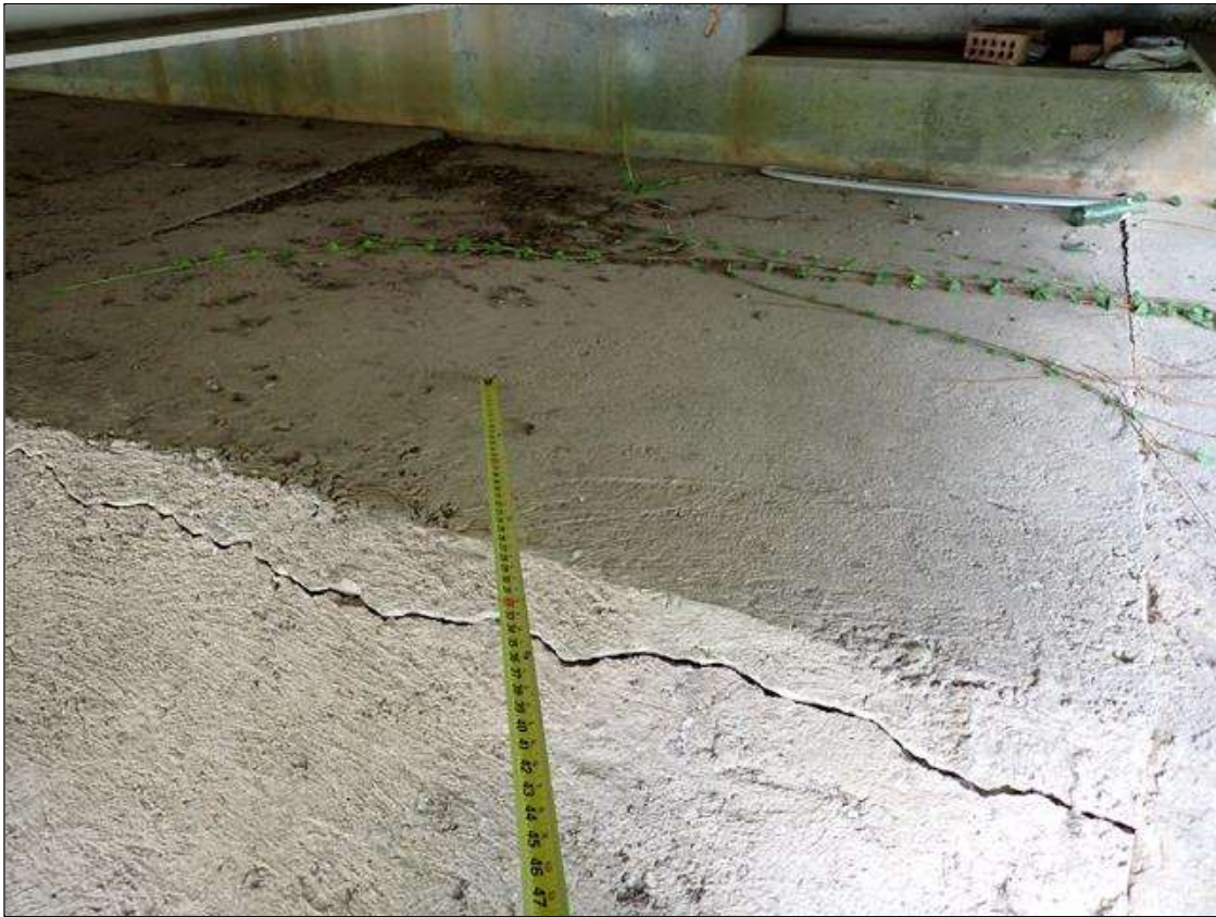
end bent 2 slope protection, below bays 3 and 4, adjacent to end bent, settlement (up to 1.5 inch deep) with transverse crack (1/4 inch x 8 feet)
