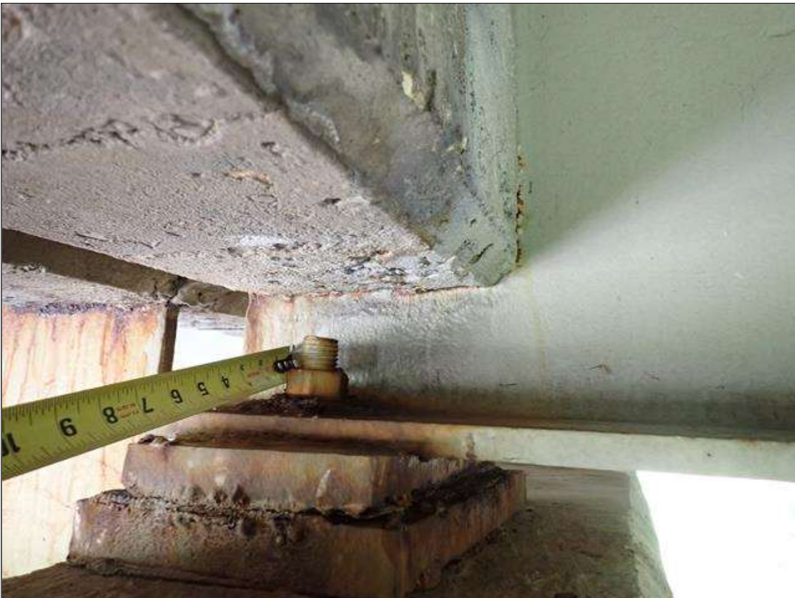
Span 1 Beam 2: at bent 1, web adjacent to diaphragm, painted over section loss (7/16 inch average remaining x 9 inch x 1 inch) with adjacent pitting (up to 1/8 inch deep) with corrosion reinitiated
