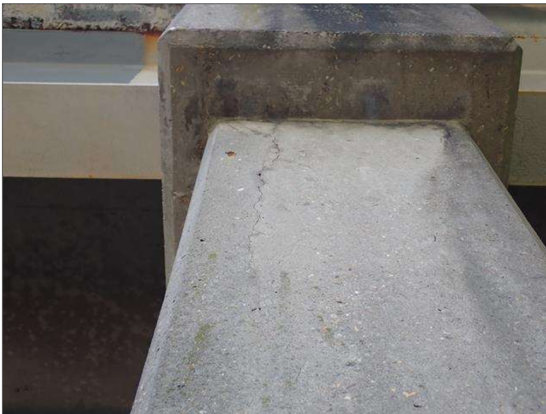
Bent 1 Pile 1: northwest corner, adjacent to cap, delamination (2.5 feet x 6 inch) with cracks (up to 1/32 inch)
