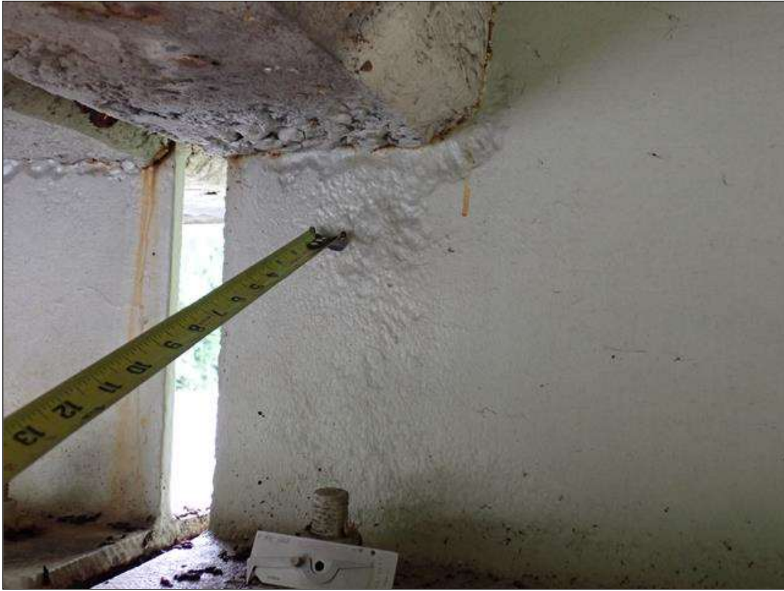
Span 4 Beam 1: (PAR) at bent 3, web adjacent to diaphragm, painted over section loss (7/16 inch average remaining x 8 inch x 4 inch)
