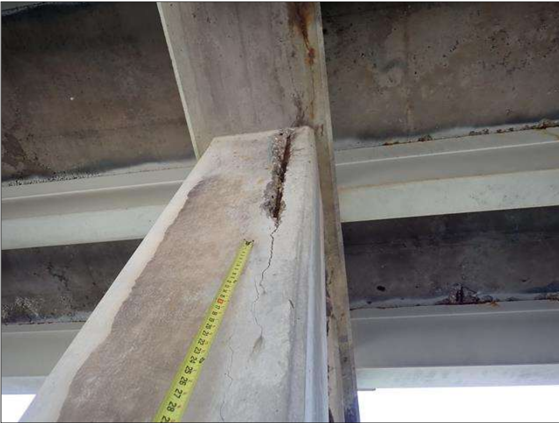
Bent 2 Pile 5: (PAR) west and east faces, near cap, spalls/delaminations (6 feet x 6 inch x 2 inches deep) with cracks (up to 1/8 inch); H-pile flange exposed with rust scale
