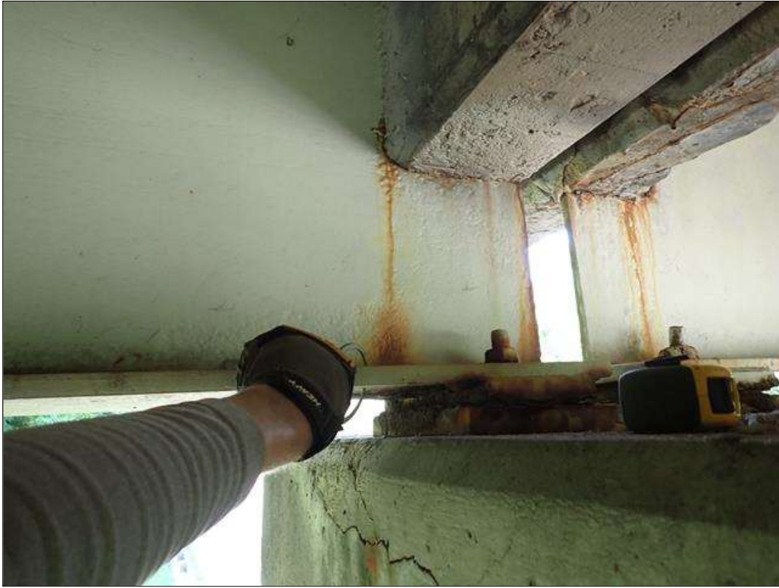
Span 1 Beam 1: at bent 1, painted over section loss: web adjacent to diaphragm (1/2 inch average remaining x 6 inch x 3 inch), lower web (1/2 inch average remaining x 13 inch x 4 inch) with corrosion reinitiated; bottom flange, corrosion with section loss (0.85 inch average remaining x 8 inches)
