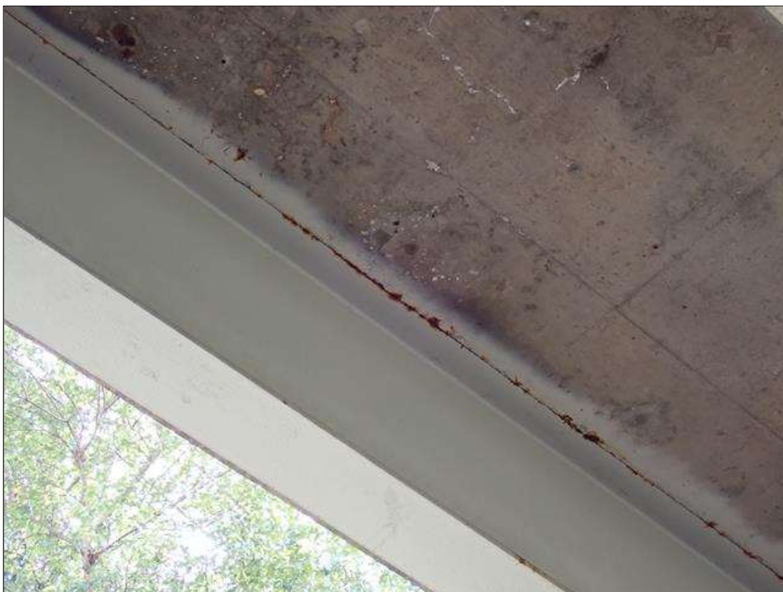
Span 1 Beam 5: along the top flange, surface rust at random
