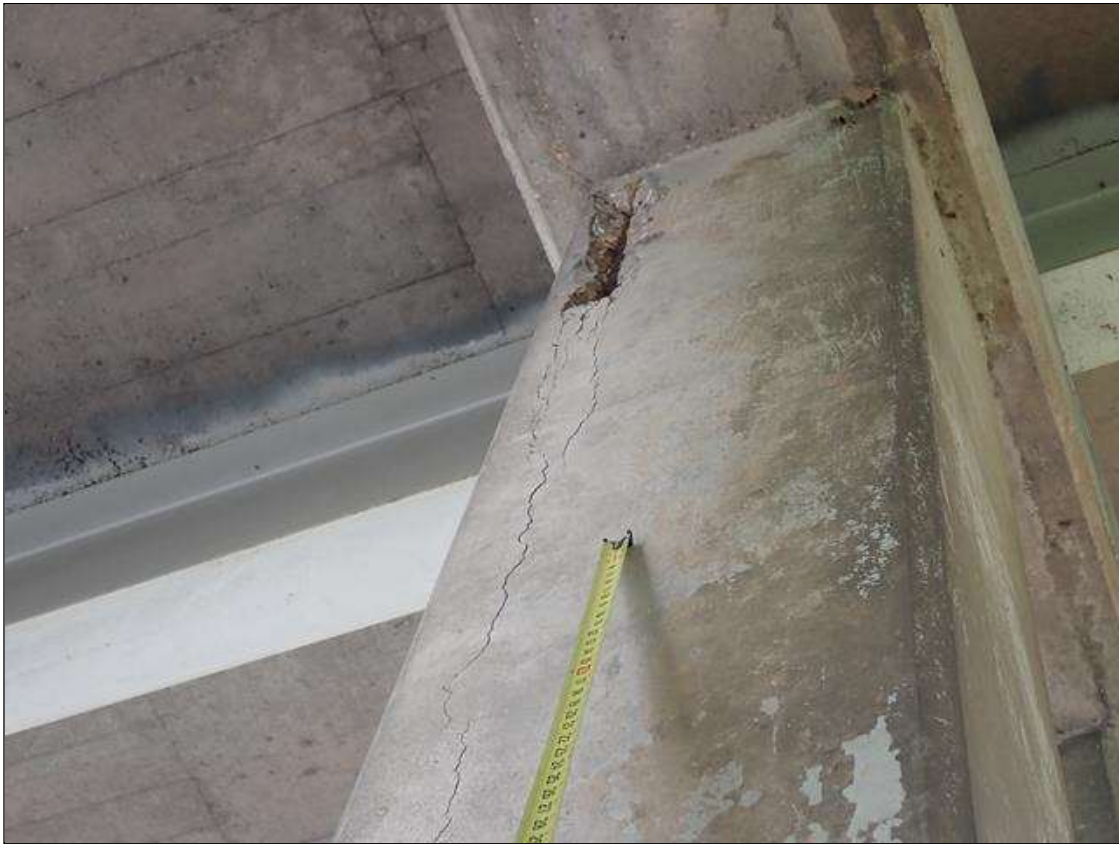
Bent 3 Pile 3: (PAR) southeast corner, near cap, spall/delamination (7 feet x 6 inch x 1.5 inch deep) with cracks (up to 1/16 inch) with east bottom flange exposed; flange has rust scale
