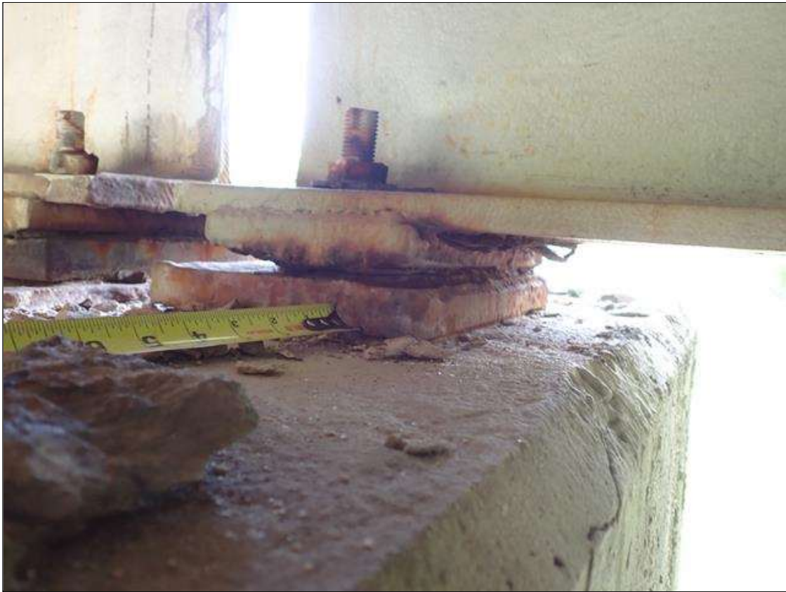
Span 1 Beam 5 - Far Bearing 5: painted over section loss (up to 3/16 inch deep) with corrosion reinitiated; pack rust
