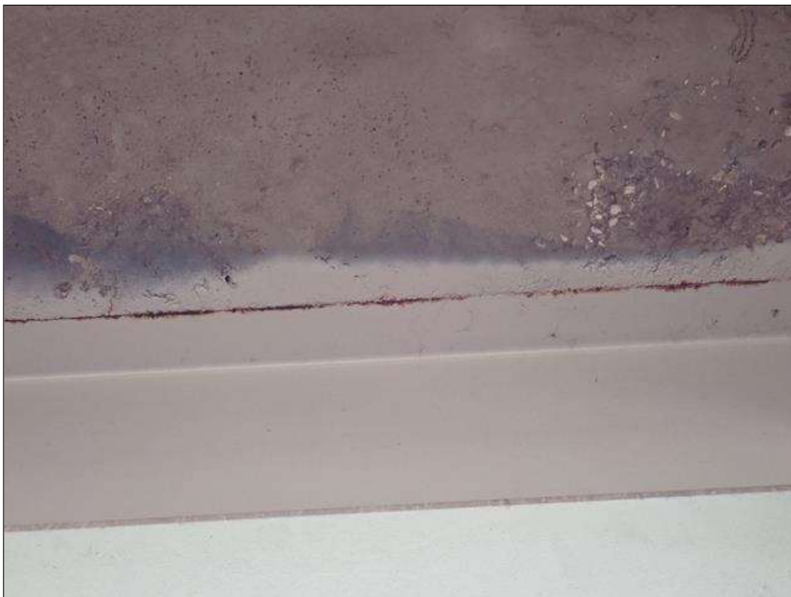
Span 4 Beam 5: along the top flange, surface rust at random
