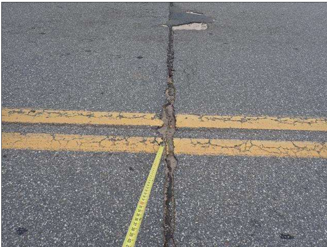
Span 4 Expansion Joint 3: along the length of the joint, areas of deteriorated seal
