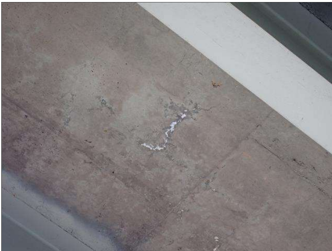
Span 4 Deck: (PAR) UP TO 1/32 INCH MAP CRACKING BOTTOM OF DECK some with efflorescence and rust stain
