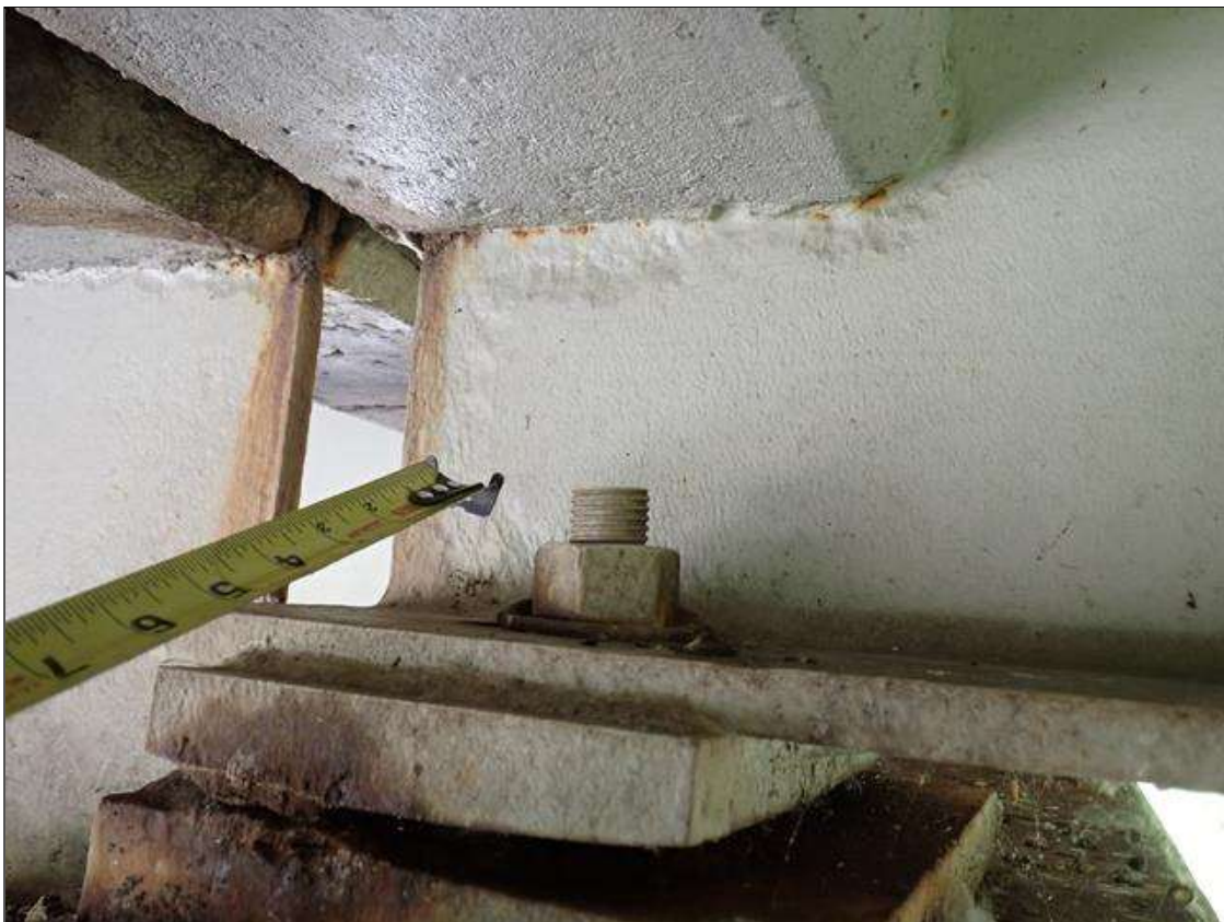
Span 4 Beam 4: (PAR) at bent 3, painted over section loss: web adjacent to diaphragm (3/8 inch average remaining x 9 inch x 1.5 inches); lower web (7/16 inch average remaining x 4 inch x 2 inch) with corrosion reinitiated
