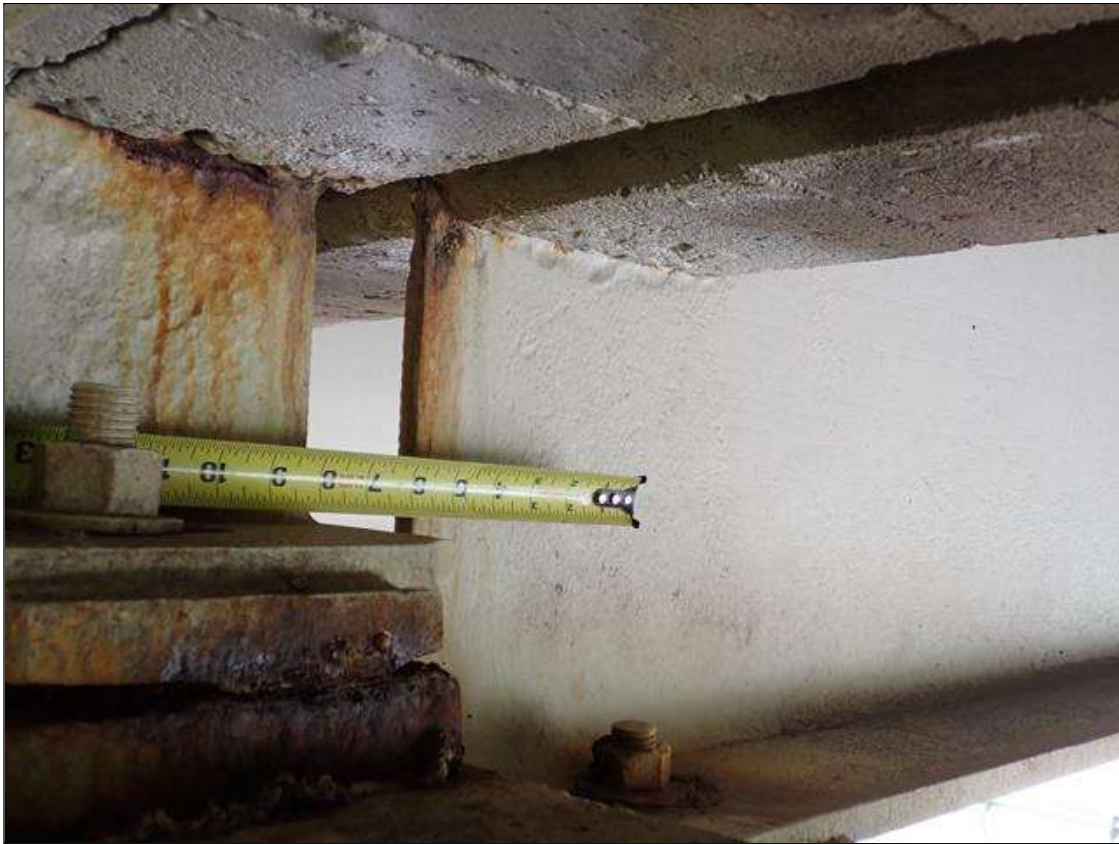
Span 3 Beam 3: (PAR) at bent 3, web adjacent to diaphragm, painted over section loss (7/16 inch average remaining x 10 inch x 2 inch) with corrosion reinitiated
