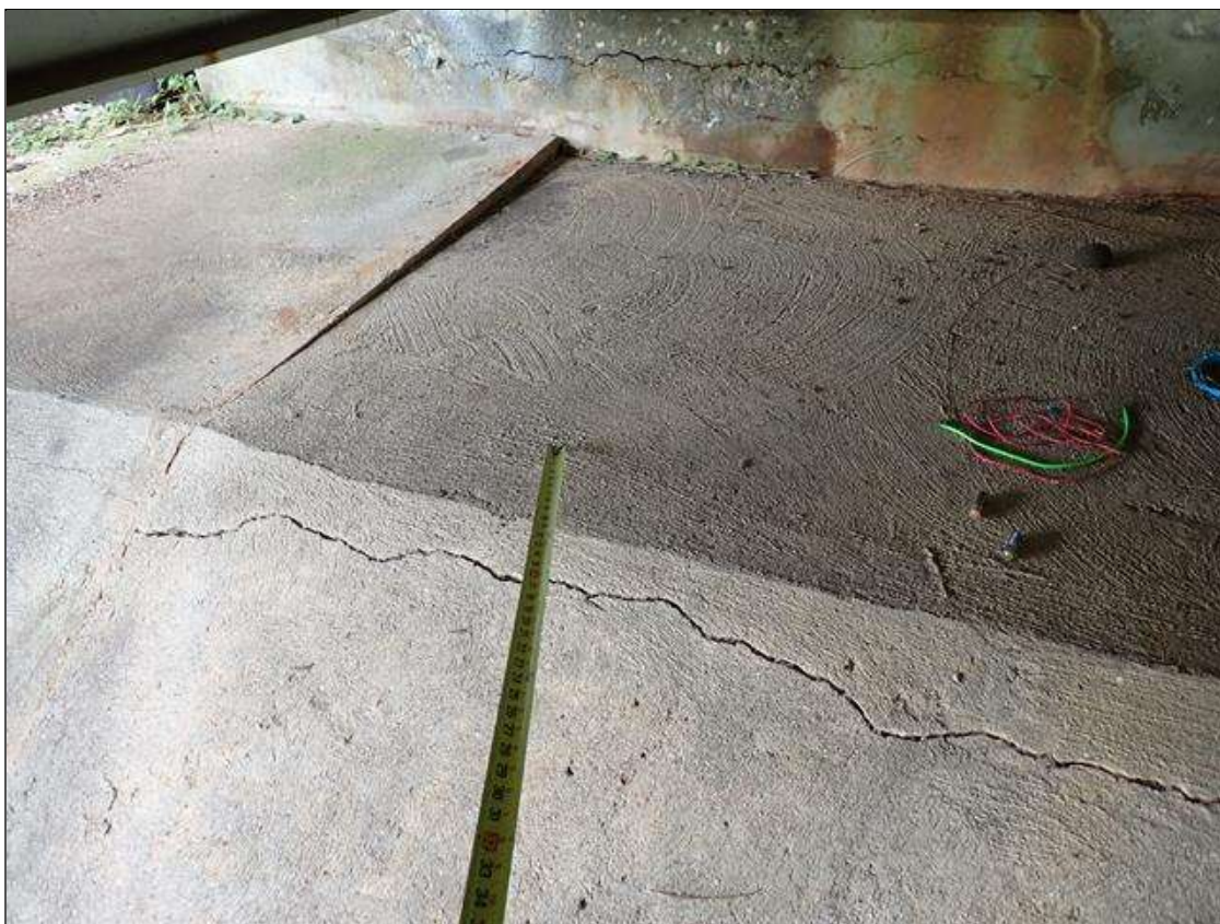
end bent 1 slope protection, below all bays, settlement (up to 2 inches) with longitudinal crack (1/4 inch x 8 feet)
