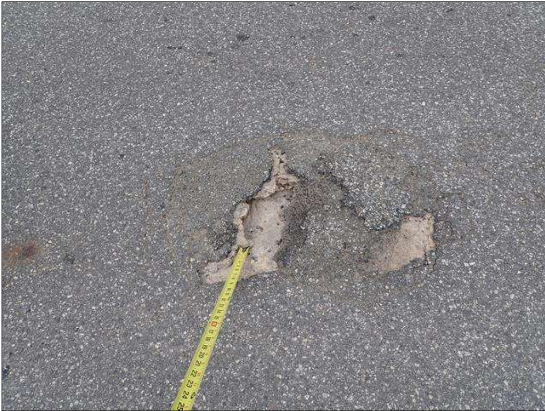
Span 3 Deck: (PAR) top of deck, in northbound lane, at areas of missing asphalt, spalls/delaminations (up to 27 inch x 2 feet x 1.5 inch deep), some with exposed rusted rebar
