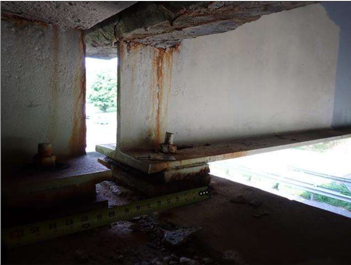
Span 2 Beam 1: at bent 1, web adjacent to diaphragm, painted over section loss (1/2 inch average remaining x 4 inch x 5 inch); bottom flange, painted over pitting (up to 1/8 inch deep x 1.5 feet) with corrosion reinitiated
