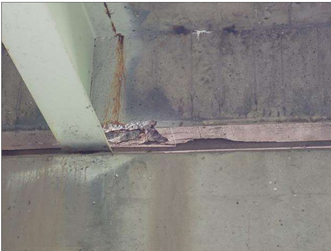
Span 1 Deck: at bent 1, bay 3 end diaphragm, spall/delamination (2.5 feet x 8 inch x 2 inches deep) with exposed rusted rebar
