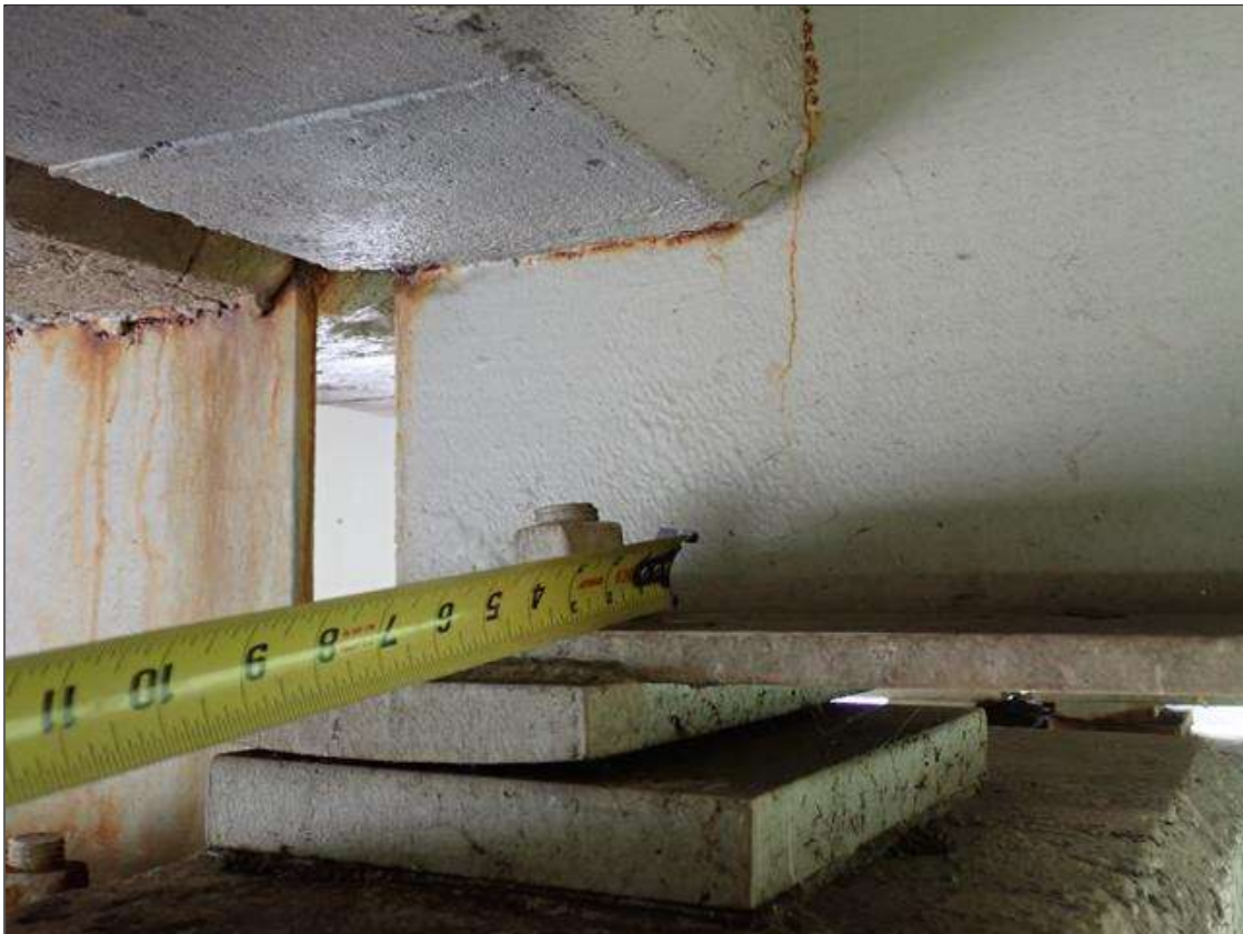
Span 4 Beam 2: (PAR) at bent 3, web adjacent to diaphragm, painted over section loss (3/8 inch average remaining x 3 inch x 1 inch) with corrosion reinitiated
