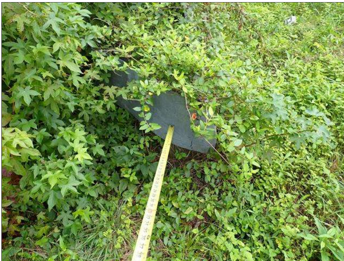
(PAR) southwest guardrail termination, impact damage (1 foot)
