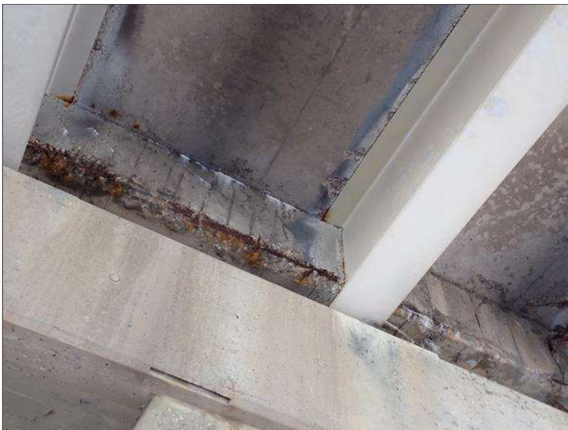
Span 2 Deck: at bent 1, end diaphragm in all bays, spalls/delaminations (up to full bay width x 8 inch wide x 2 inches deep) with exposed rusted rebar with cracks (up to 1/16 inch) with efflorescence
