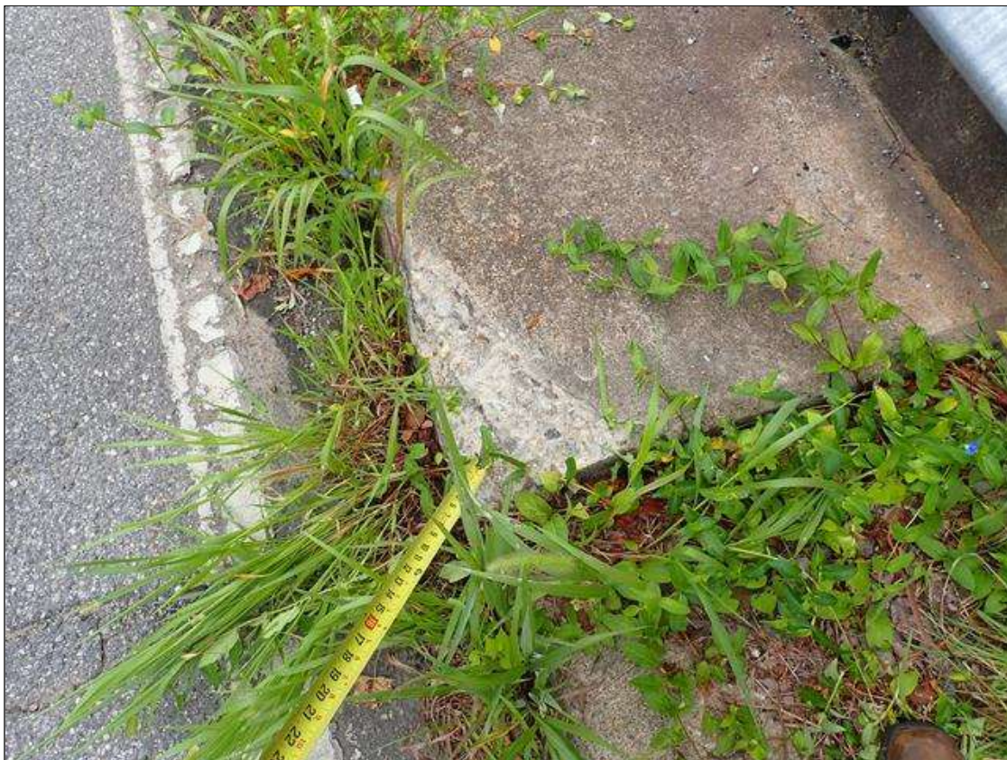
Span 1 Right Bridge Rail: at corner of sidewalk adjacent to end bent 1, spall [18 inch x 10 inch x 4 inch deep] no exposed rusted reinforcing
