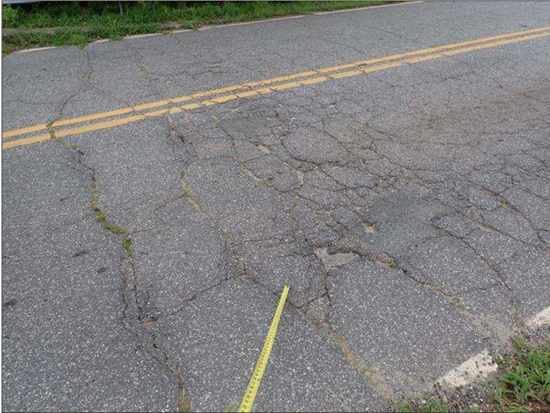
south and north approach asphalt, broken asphalt with cracks (up to 1 inch wide) and spalls (up to 8 inch diameter x 1.5 inch deep); settled (up to 1 inch) in relation to bridge
