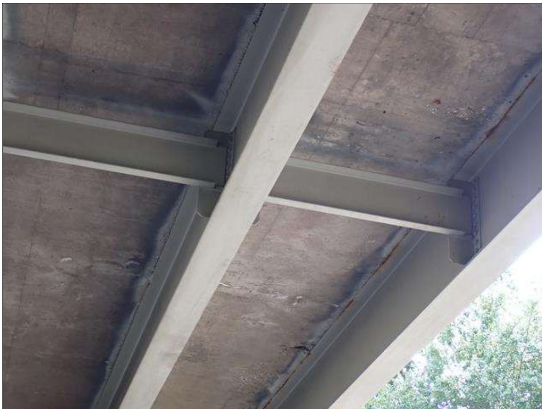
Span 3 Deck: (PAR) BOTTOM OF DECK UP TO 1/32 INCH MAP CRACKING AT RANDOM THROUGHOUT SOME WITH EFFLORESCENCE AND RUST STAINS
