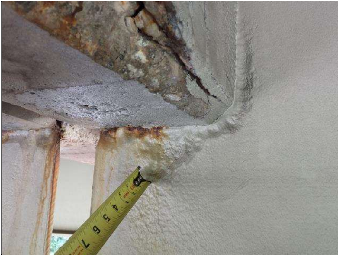
Span 3 Beam 3: (PAR) at bent 2, web adjacent to diaphragm, painted over section loss (3/8 inch average remaining x 10 inch x up to 10 inch), with adjacent pitting (up to 1/8 inch deep), with corrosion reinitiated
