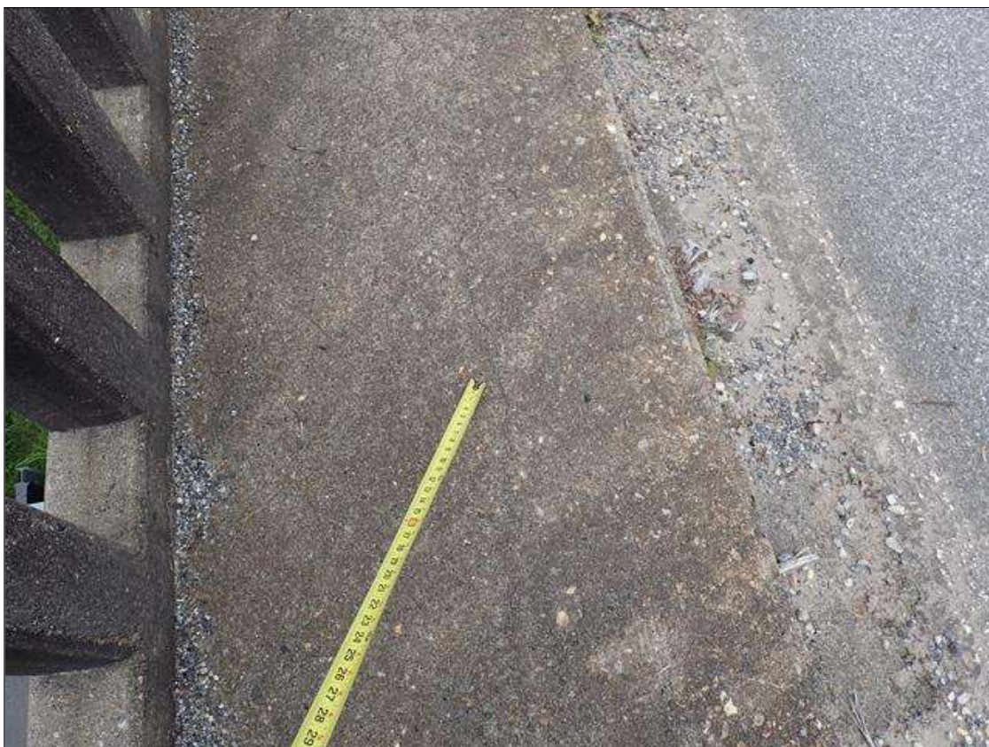
Span 2 Right Bridge Rail: sidewalk near bent 1, longitudinal/map cracks (up to 1/32 inch)
