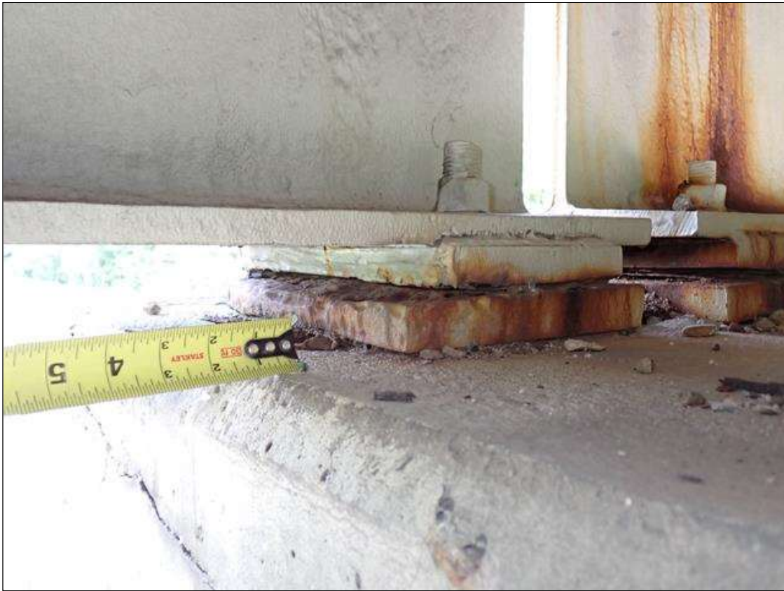
Span 3 Beam 5 - Near Bearing 5: painted over section loss (up to 3/16 inch deep) with corrosion reinitiated; pack rust
