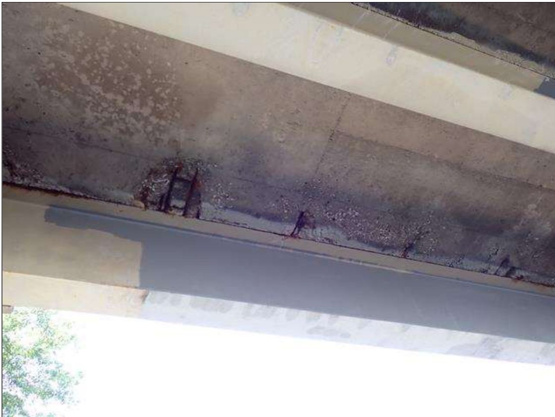
Span 2 Deck: (PAR) underside of bays 1 and 4, and left overhangs at bent 2, spalls/delaminations (up to 2.5 feet x 2 feet x 3 inches deep) with exposed rusted rebar; rebar has approximately 10 percent section loss
