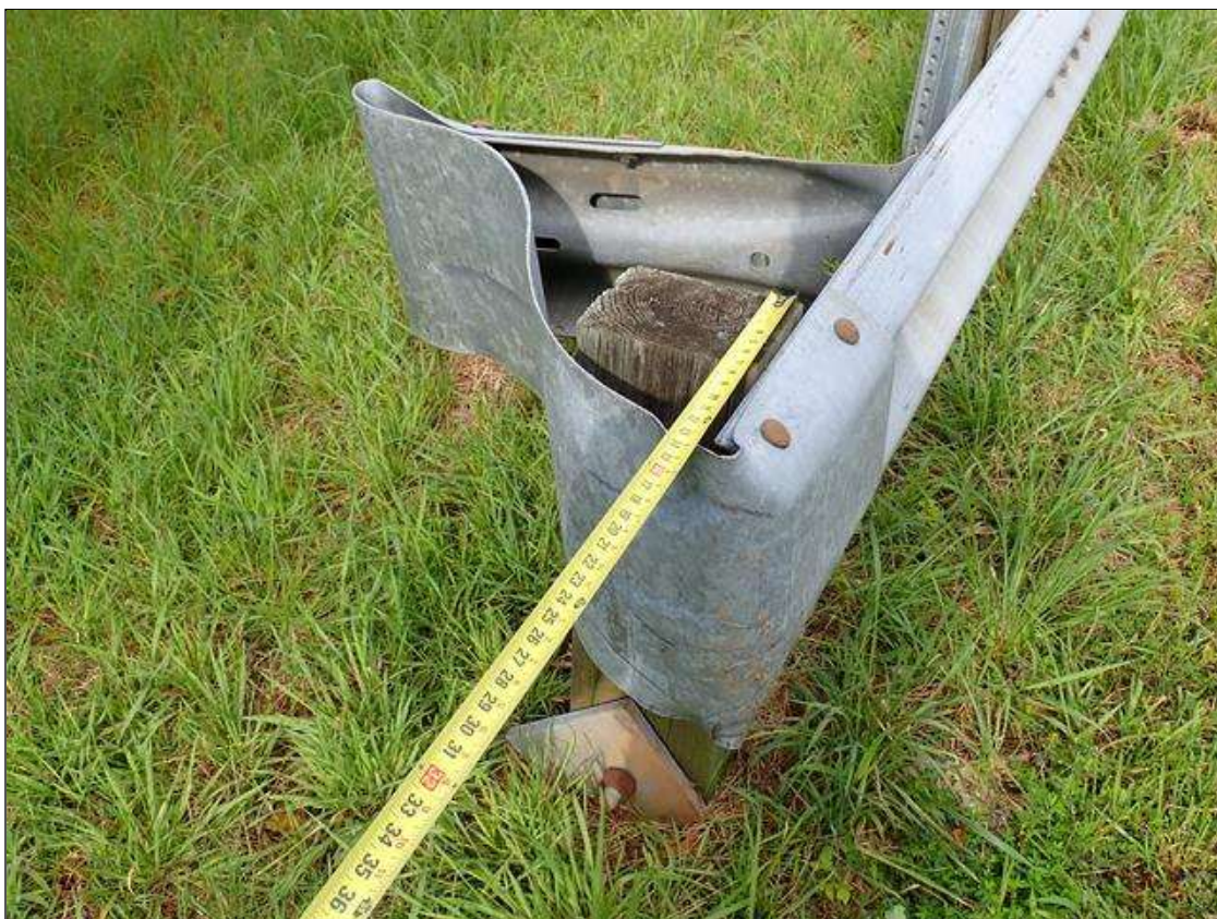
(PAR) northeast guardrail termination, impact damage (1 foot)
