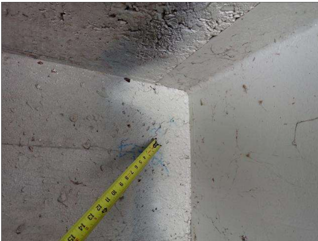
End Bent 2 Abutment: up to 8 INCH x UP TO 1/32 INCH VERTICAL AND DIAGONAL CRACKS AT BEAM ENDS
